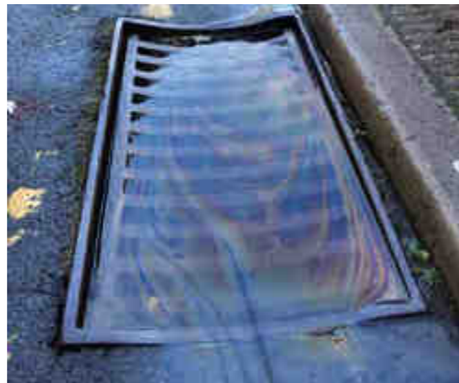
Pollution from roads and car parks is often visible - fuels, oil, heavy metals, tyre dust and silt all get washed into drainage systems.
