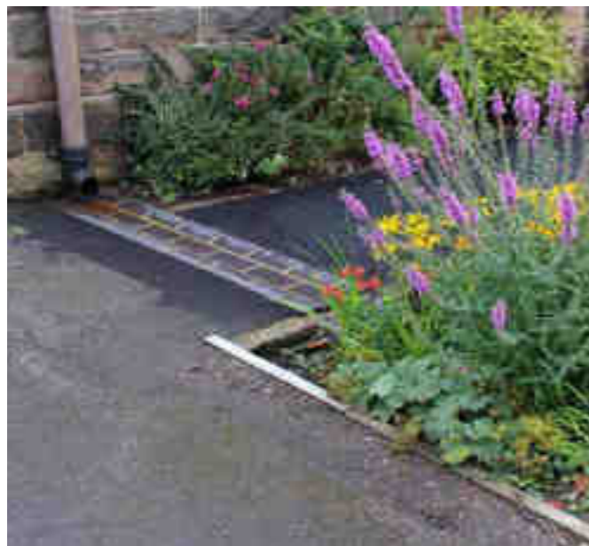
Strutts Centre, Belper. A retrofit downpipe shoe and brick channel into a raingarden.
