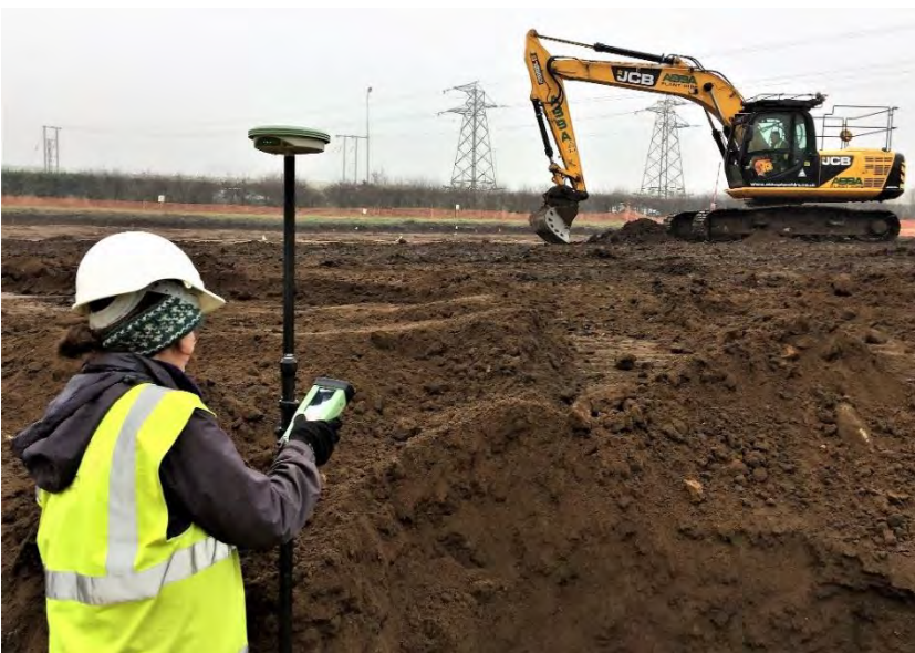
Plate 14: Mechanical topsoil stripping over Roman 'villa' site; DGPS survey in left foreground
